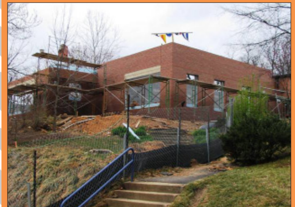
Mount Daniel Elementary School's addition is well underway, and proceeding according to schedule.
